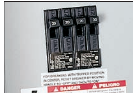
circuit breakers six 20-amp branch breakers provide protection for the external loads
